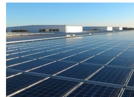
Solar Power Generation Panels (Ibaraki Nishi Distribution Center)
